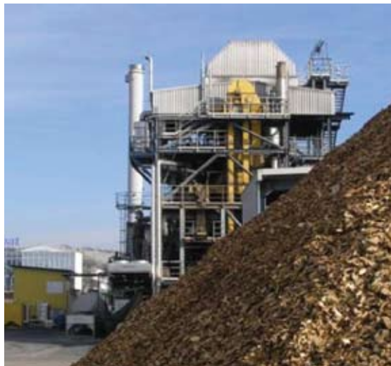
Figure 4. Fluidized Bed Gasifier in Güssing (Burgenland, Austria)
